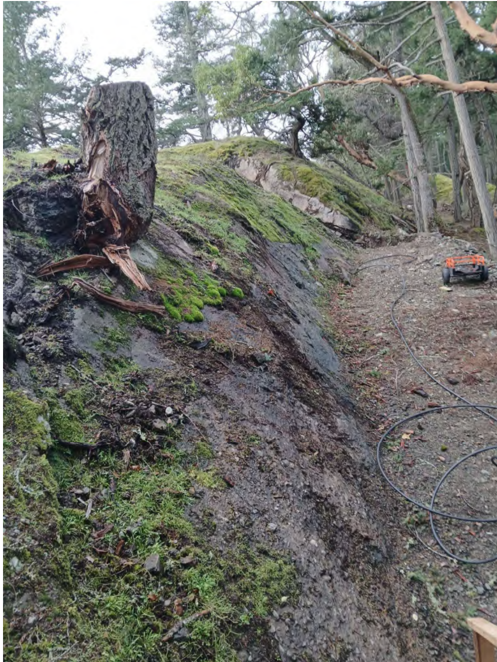
Plate 2. Loss of herbaceous cover from the bedrock surface in the Herbaceous Ecosystem DPA due to construction of utilities access corridor at 6915 Pirates Road, Pender Island, BC. Also visible is the felled veteran Douglas-fir stump at the top of the ridge.
