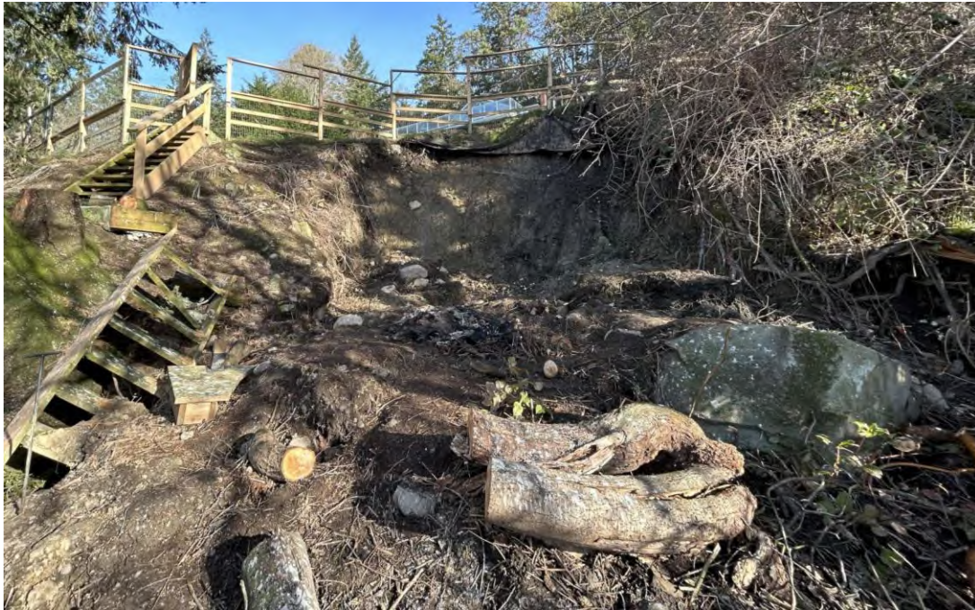
Photo 1: Standing near shoreline looking NW at landslide. Note soft soil and other debris in foreground.
