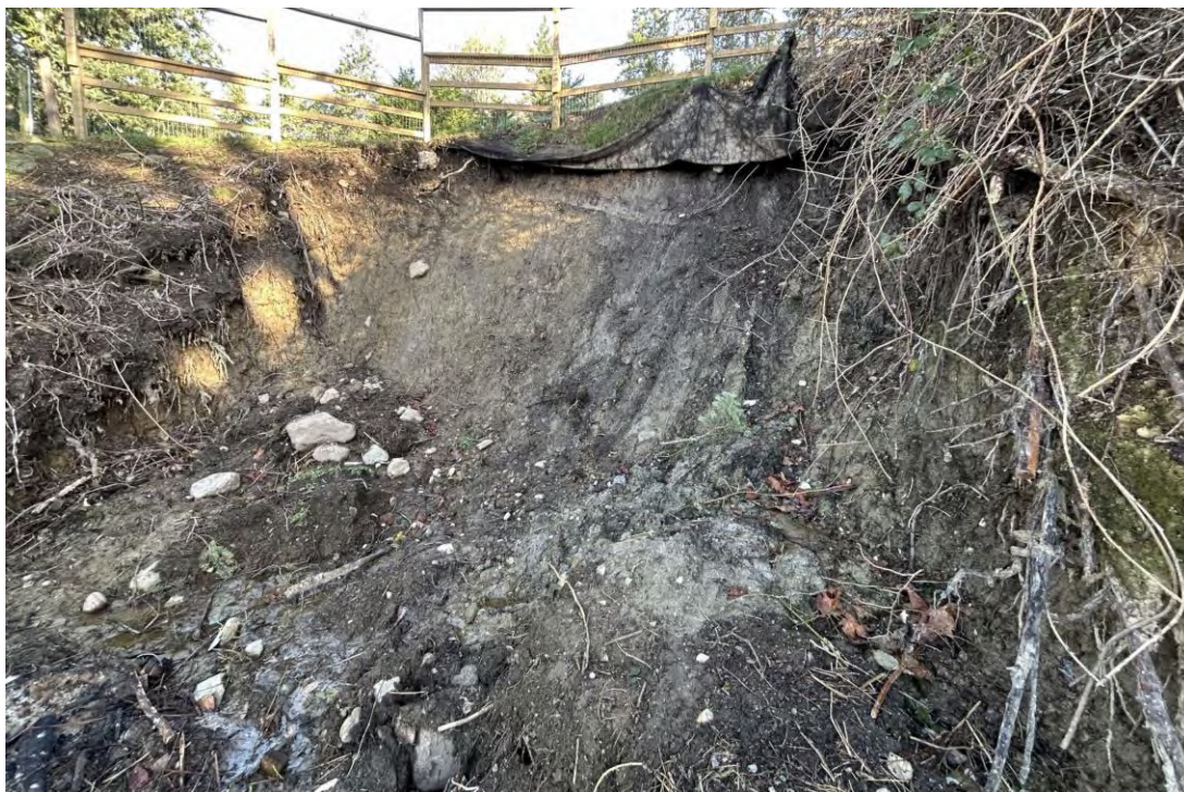
Photo 2: Closeup of landslide scarp.
