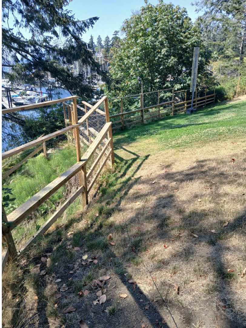
Plate 1. Fenced grassy area above localized erosion slump at 2319 MacKinnon Road.
