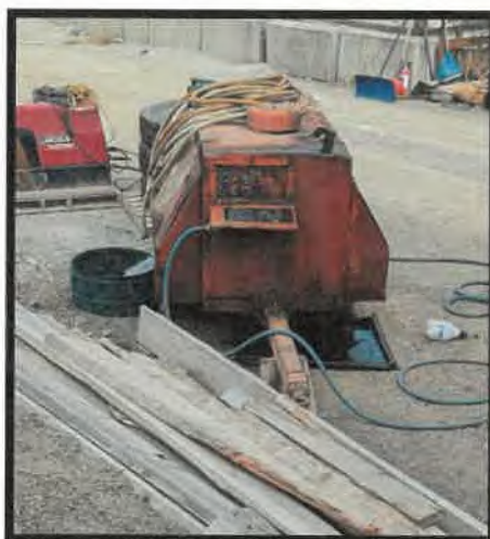
Photo 18: Drip tray noted below compressor.
