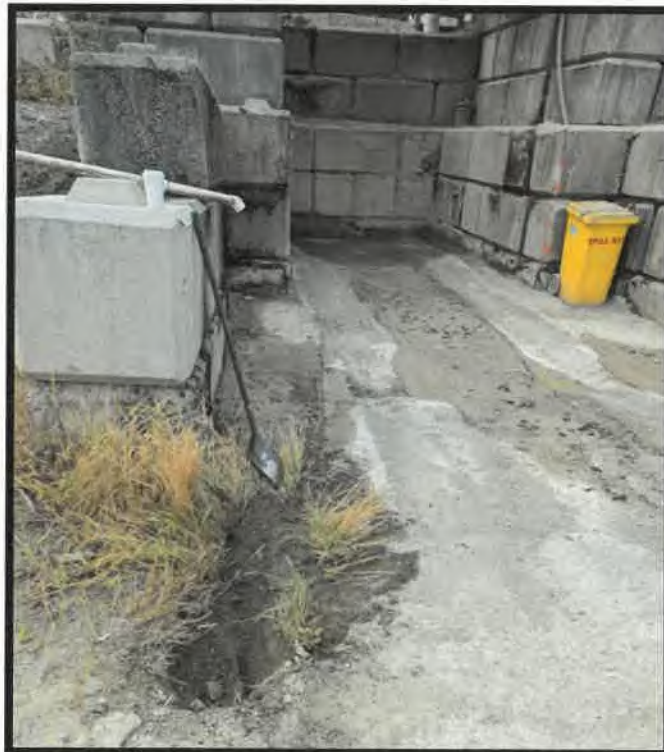
Photo 6: Batching area, requires maintenance to ensure drainage is not blocked.
