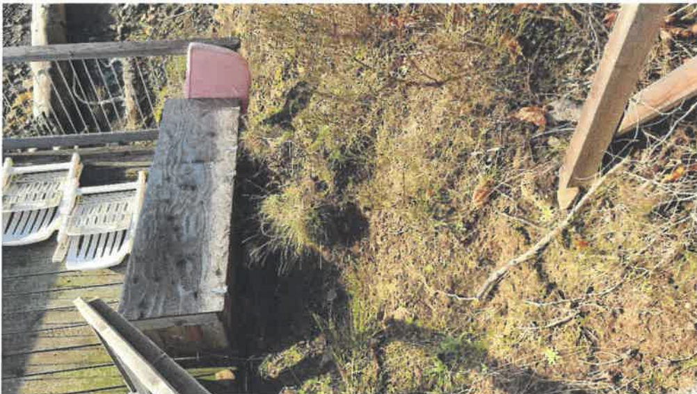
Photo 8: Area directly above deck is susceptible to soil disturbance and erosion.
