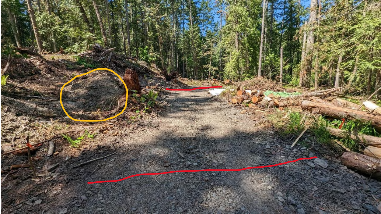
Photo 9 shows the portion of the driveway within the DPA that was added and extended from the original pre-existing driveway, between the red lines. Topsoil that was removed from the new road section is stored off to the side, outlined in yellow.
