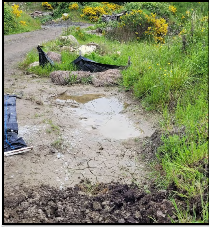
Photo 11 – Sediment buildup adjacent to silt fencing up-gradient of settling pond. It is recommended that ditching is excavated on a regular basis to avoid over sedimentation and rerouting of surface runoff.
