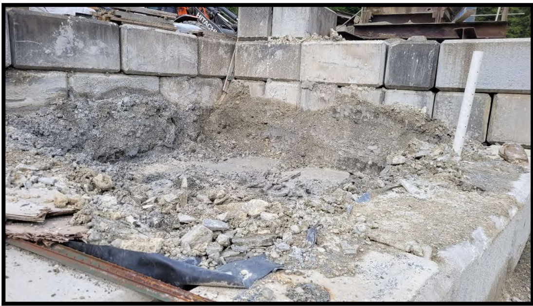
Photo 12 – Excess concrete from cleaning of drums. Recommended to maintain minimum volume in this cell to avoid overflow / flooding.
