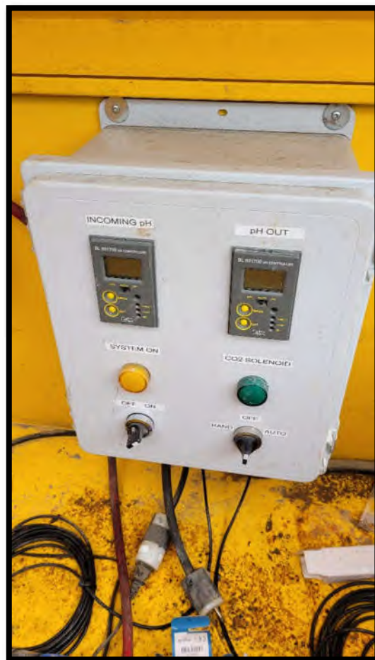
Photo 10 – Automated pH treatment controller.
