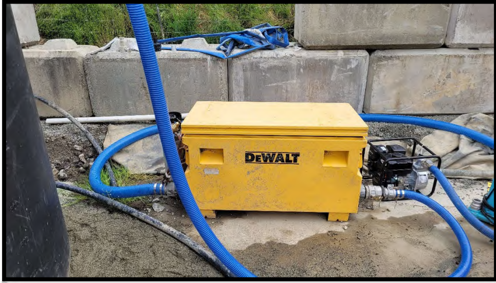
Photo 9 – Water treatment module including pH treatment.
