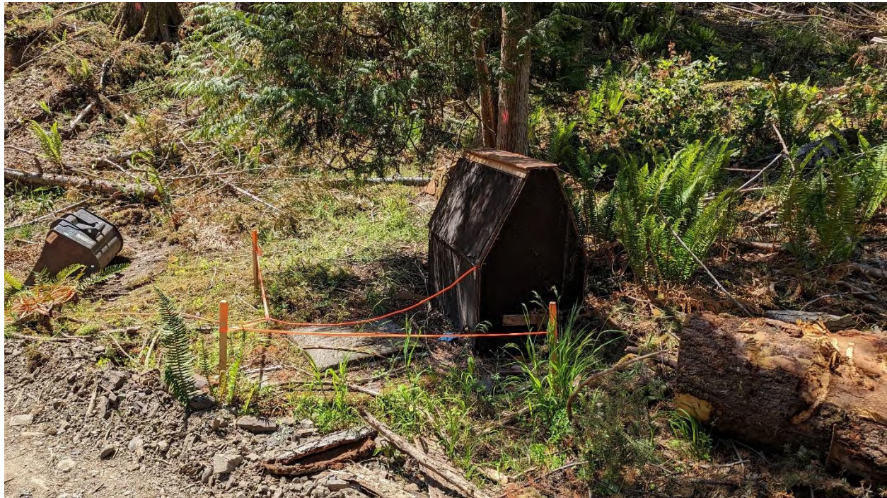
Photo 8 shows the pre-existing dug well and location for a future pump house (<100ft 2 ).
