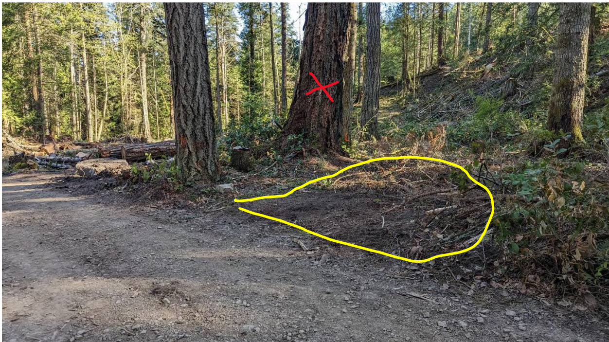
Photo 12 shows the partially compacted and temporary gravel storage site (gravel not in this photo taken on April 27th, but observed during the May 27th site visit), outlined in yellow. The cabin is just out of the frame on the left. The subject Douglas-fir is marked with a red X.
