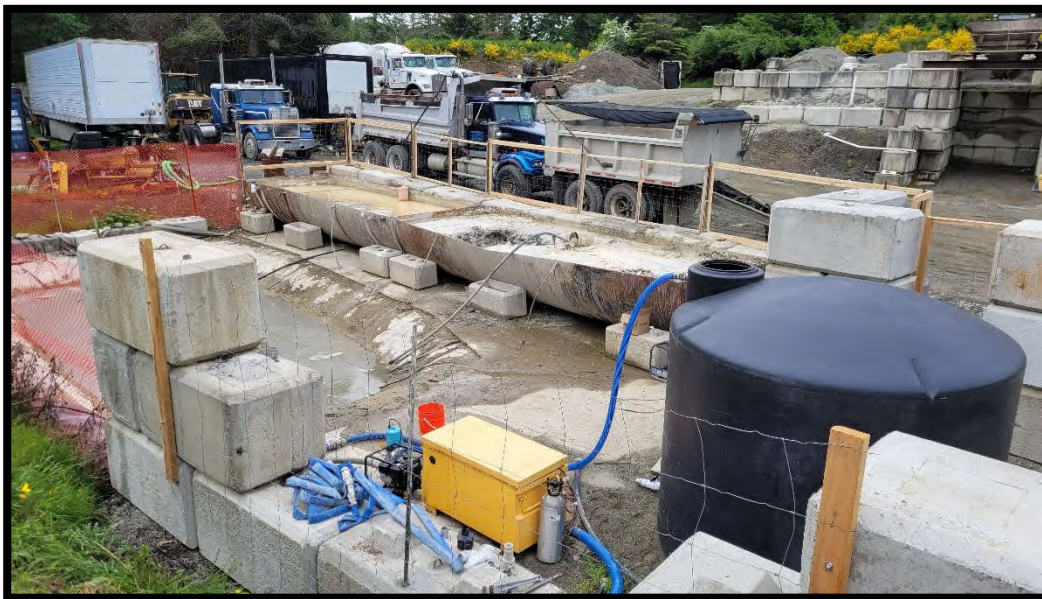
Photo 16 – Water treatment area overview.
