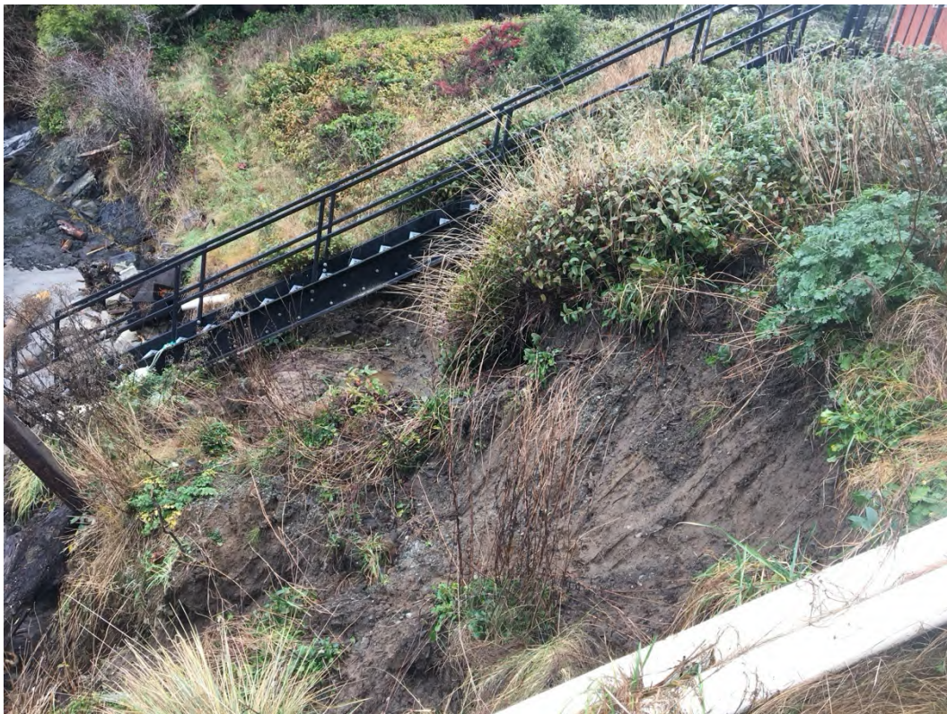
Photo 10. Eroding slope - additional soil slippage has occurred in winter 2024/2025 (March 2025).
