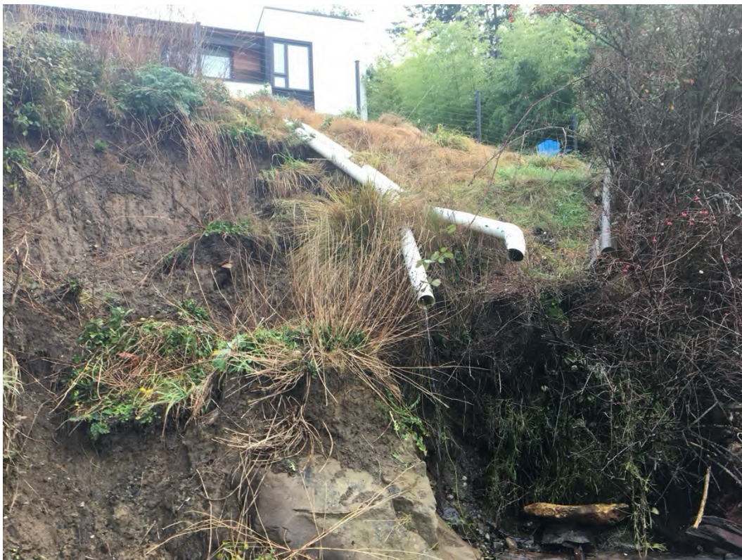
Photo 12. Eroding slope - additional soil slippage has occurred in winter 2024/2025 (March 2025), near Photo 5 location.
