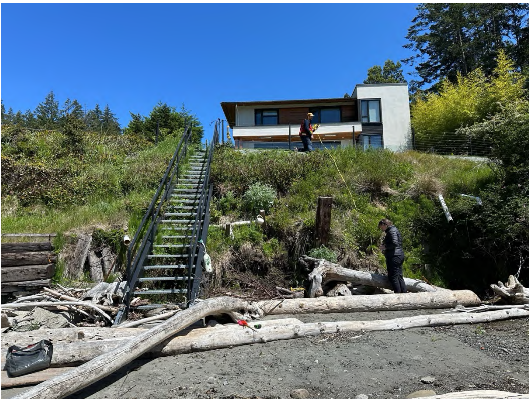
Photo 4. Looking at the shoreline and base of eroding slope (May 2024). Additional soil slippage has occurred in winter 2024/2025 – see Photos 10-12.
