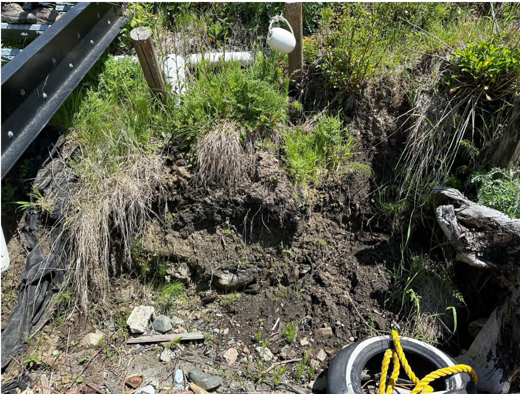
Photo 5. Erosion at base slope (May 2024). Additional soil slippage has occurred in winter 2024/2025 – see Photos 10-12.
