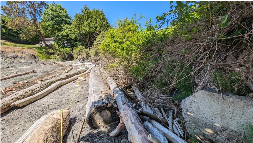
Photo 2. Looking north along the beach at the shoreline and base of eroding slope (May 2024). Additional soil slippage has occurred in winter 2024/2025 – see Photos 10-12.
