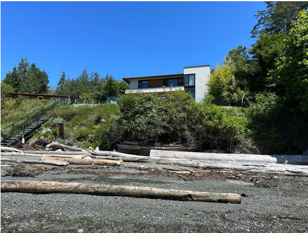
Photo 1. Looking northeast from the beach at the shoreline and eroding slope of 37149 Schooner Way (May 2024). Additional soil slippage has occurred in winter 2024/2025 – see Photos 10-12.
