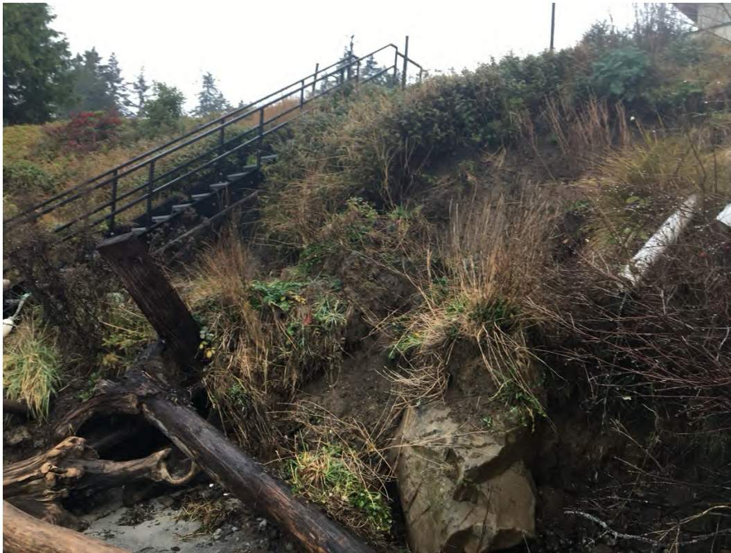
Photo 11. Eroding slope - additional soil slippage has occurred in winter 2024/2025 (March 2025).
