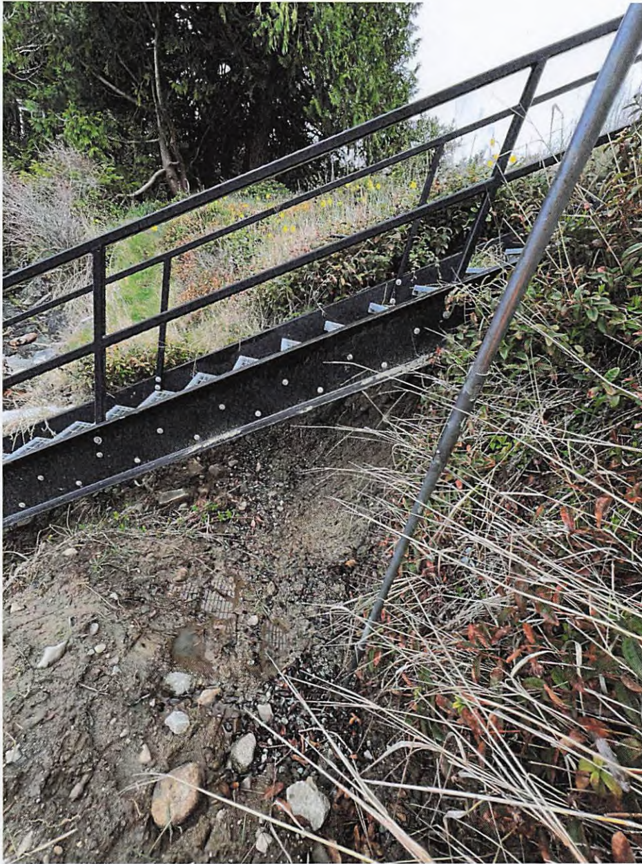
Photo 4. Soil scarp and slipped soil next to stairs. Hand auger at right indicating location of potential native sandy clay soil.
