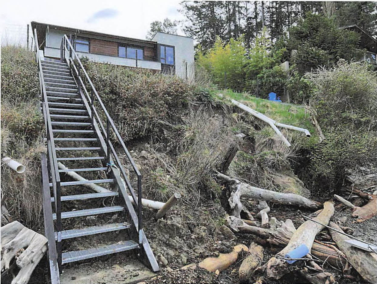
Photo 3. Stairs and recent slipped soil material and scarp.
