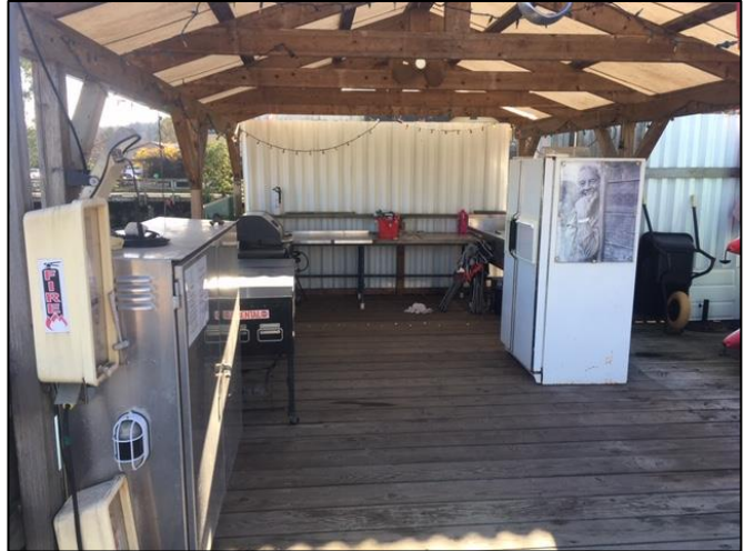
Image 6 – Filled foreshore area of subject property showing communal kitchen built on portion of Ganges Harbour boardwalk.
