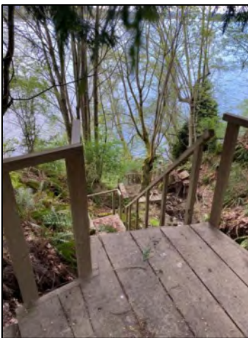
Figure 3 Existing stairs in disrepair leading to shoreline
