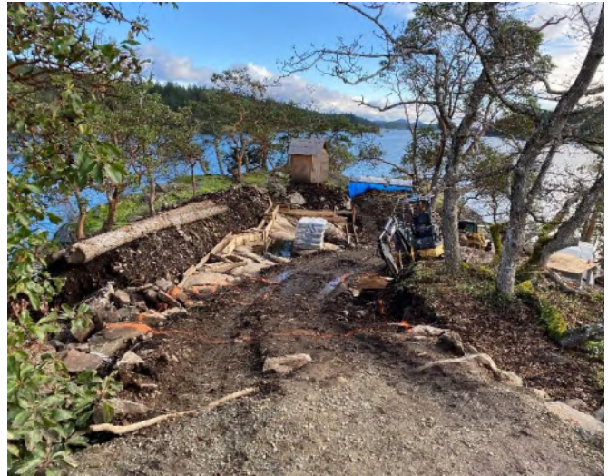
Photo 2: Soil disturbance and berming on access leading up to build site.
