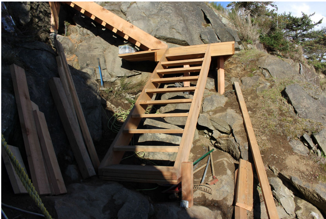
Plate 10. Disturbance to soil veneer and associated vegetation on rock bluff during stairway construction in Bluffs Ecosystem DPA at 130 Cliffside Rd., Saturna Island BC. (Photo courtesy of Glenn Fjordbotten)
