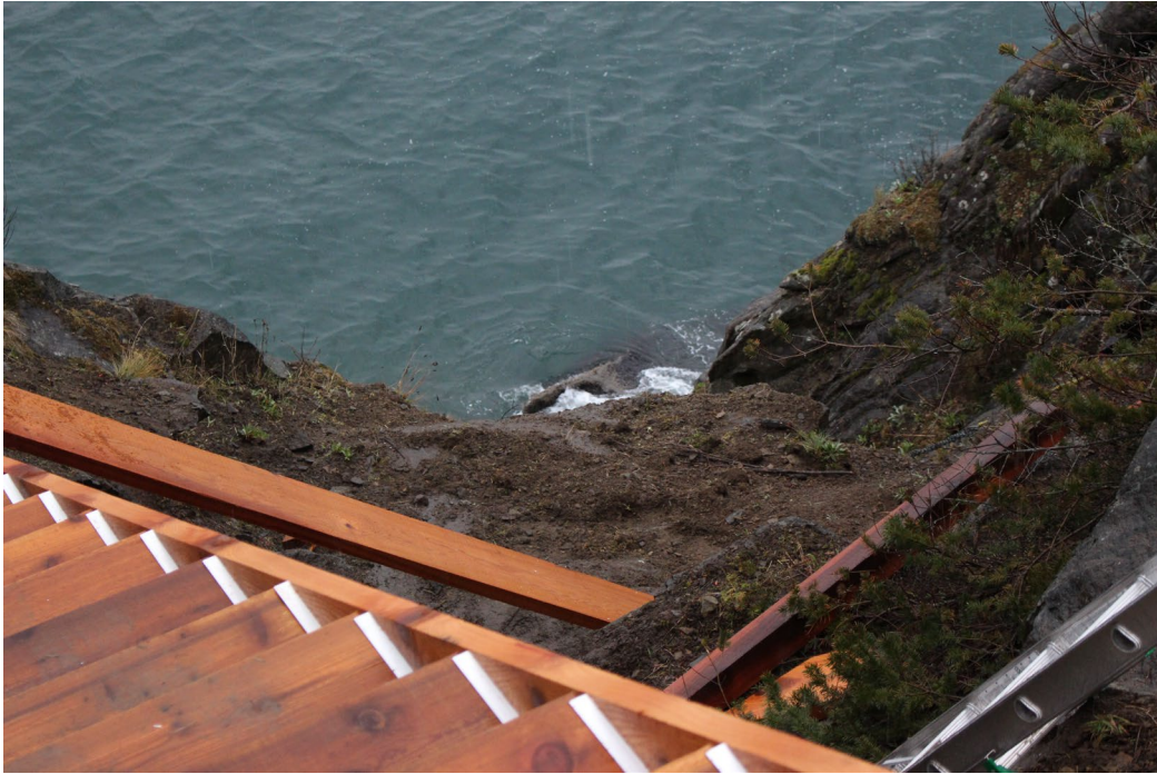
Plate 9. Disturbance to soil veneer and associated vegetation on rock bluff during stairway construction in Bluffs Ecosystem DPA at 130 Cliffside Rd., Saturna Island BC. (Photo courtesy of Glenn Fjordbotten)
