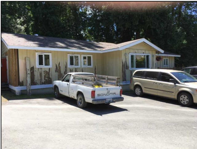
Image 7: The existing administration building was in need of refinishing at the time of staff's site visit.
