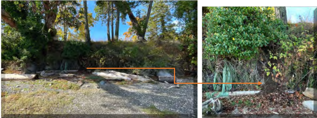
Photo #1 & #2 - E Shoreline steep repose to level of home (behind tree on left) and new septic (directly behind bank). Orange arrow points to the detritus falling from bank onto backshore area. Photo credit to D. Fenton. Oct 11, 2023.
