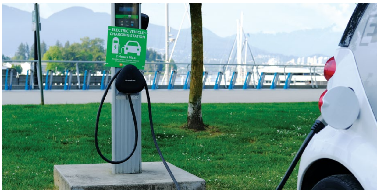
Transportation is one of the biggest sources of carbon pollution in Atl'ka7tsem/Txwnéwu7ts/Howe Sound communities. The solution is to get people out of their gas-powered cars and into electric cars, or to use more public transit and active transportation such as biking and walking. Photo: iStock
